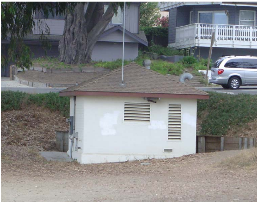
Photo 4. Lift Station Along East Cliff Drive, Santa Cruz Harbor, Santa Cruz County, California
